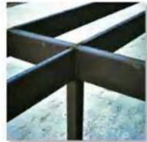
The floor beams of this building are welded together and thus form fixed connections. (10)
