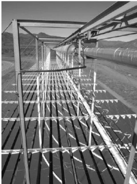
Figure 3.6 A linear Fresnel collector: in this foreground, the absorber pipe is visible; behind it is the piping with the secondary reflector (Photo DLR).
